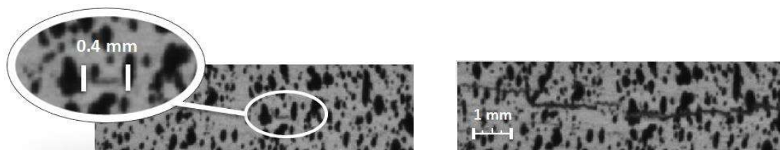
Fig. 5 Left: micro (hairline)-crack vs. Right: macro-crack (same orientation as Fig. 3)
